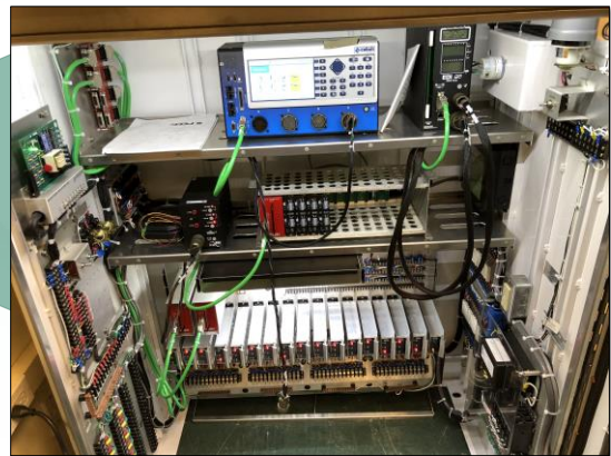
Inside of cabinet in CUTR's lab (Donated by City of Tampa)
